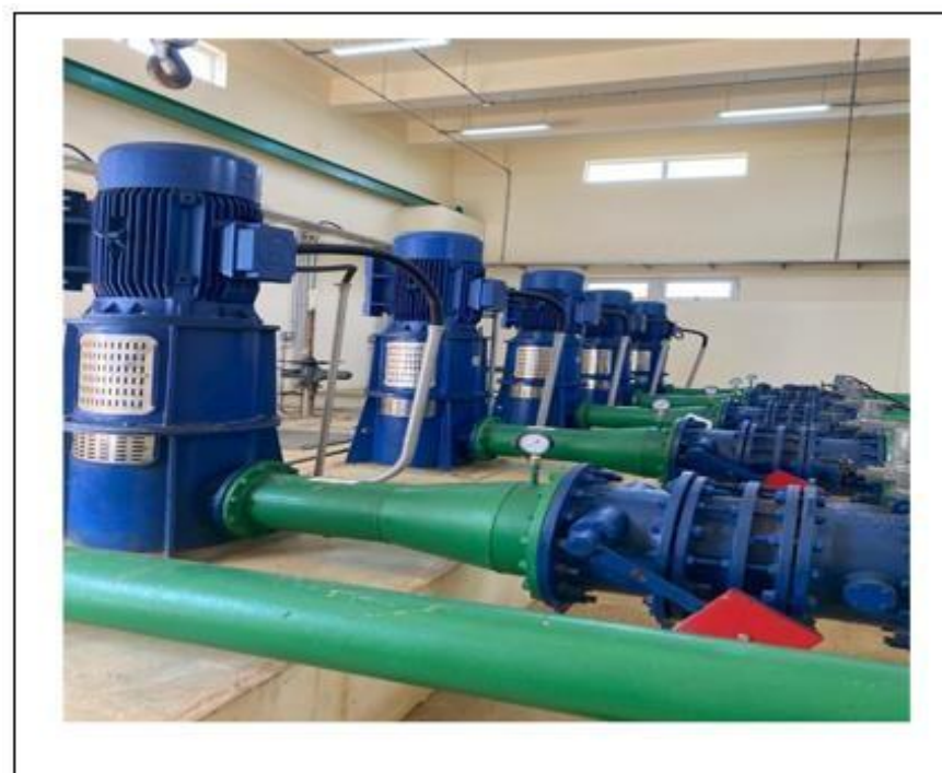
Fig 4.2 Flowmeter Chamber (low-lift section)
